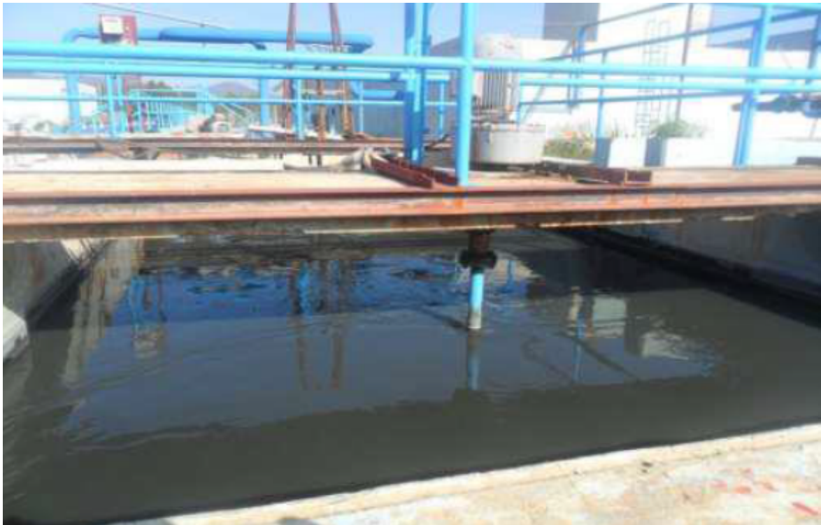
Figure 3. Mixing and neutralization basin N ° 2.
