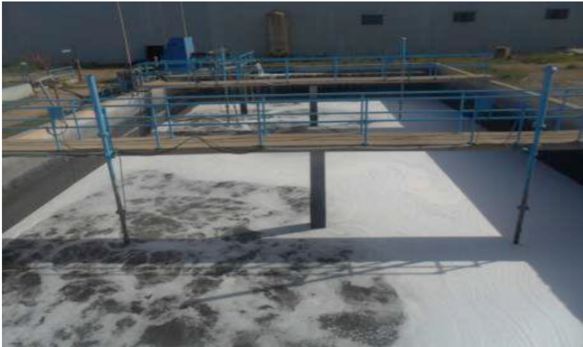
Figure 2. Photo of mixing and equalization basin N ° 1.
