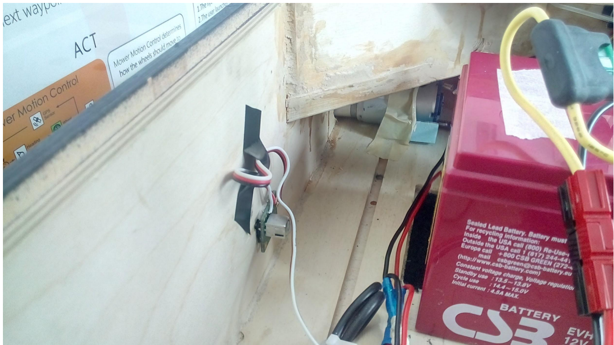
Fig 8. Difficult to service front motors.
