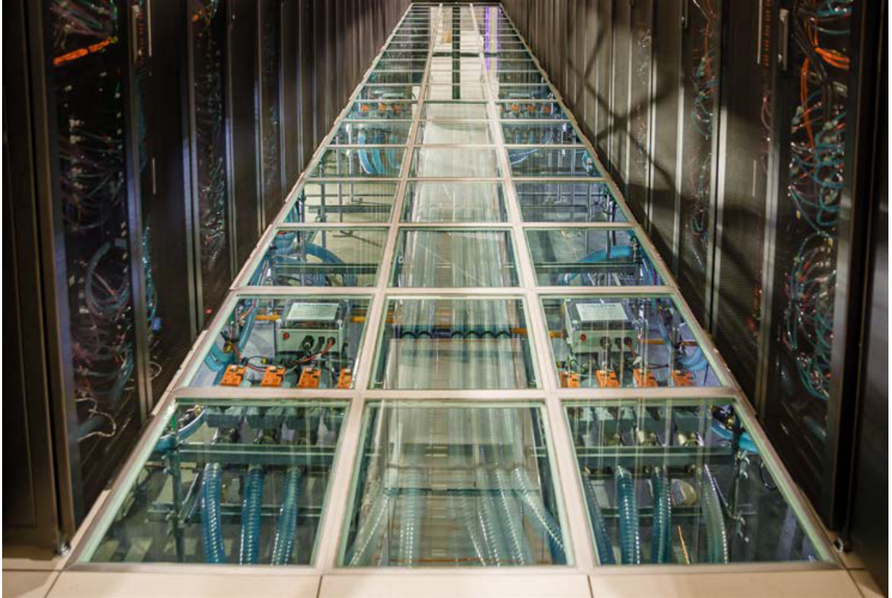
Figure 7. Sandia's liquid-cooled Attaway HPC system
