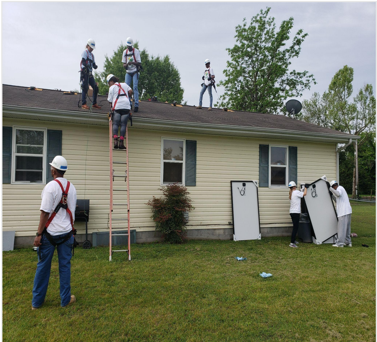
Habitat solar installation in Illinois ( photo courtesy of Aur Beck ).
