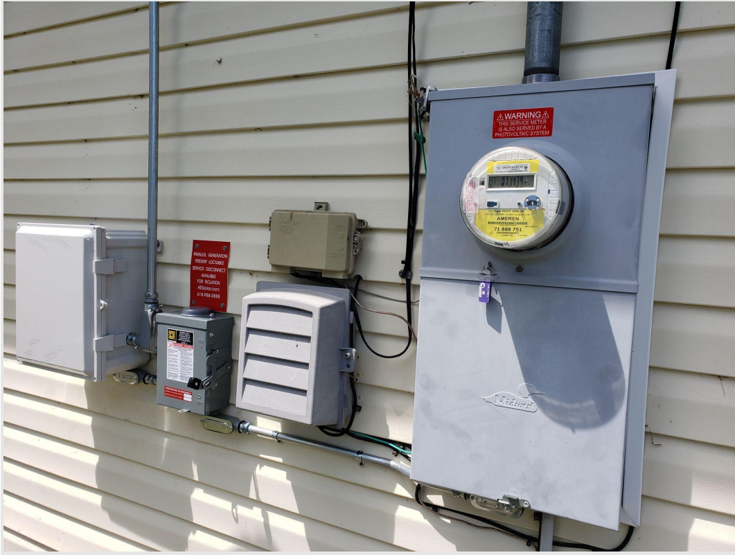
Habitat solar installation in Illinois ( photo courtesy of Aur Beck ).
