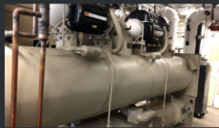
Chiller Operational Logs, Maintenance Sheets, And E Book
