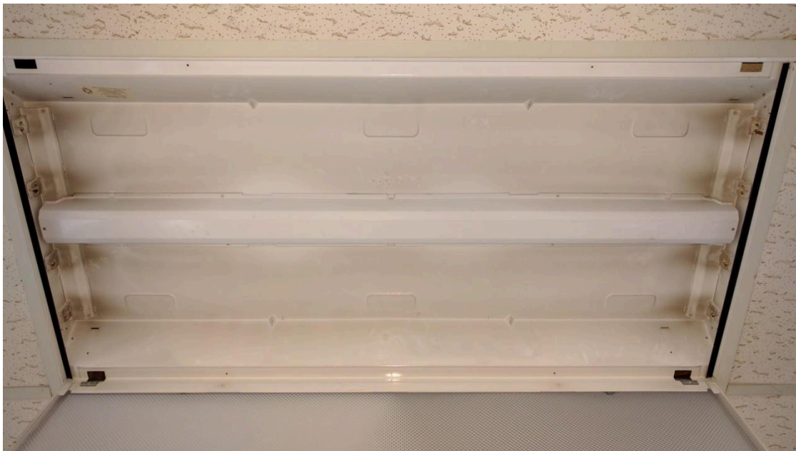
Fixture with lamps removed
