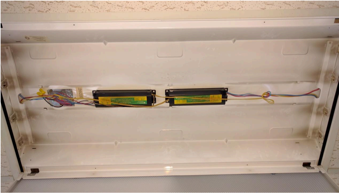
Fixture with ballast cover removed
