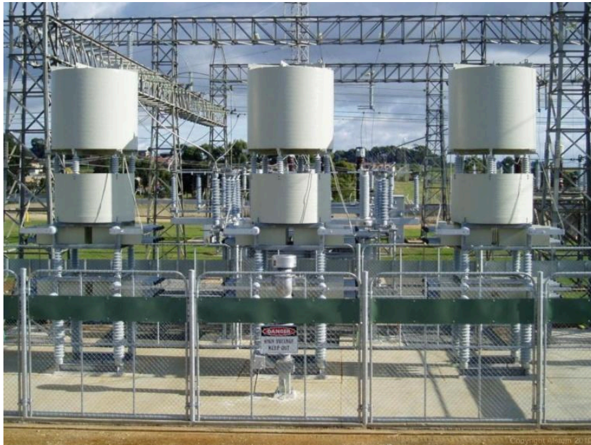
Figure 16.3 A: Harmonic Filter Banks
