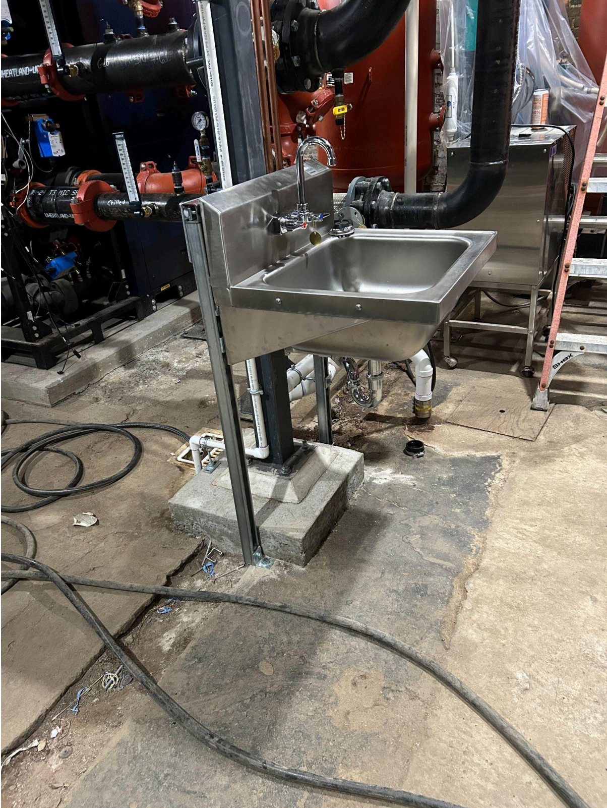
A sink that has been installed in the boiler room, so that the BSD staff has access to wash up after they have performed any maintenance in the Boiler room.
