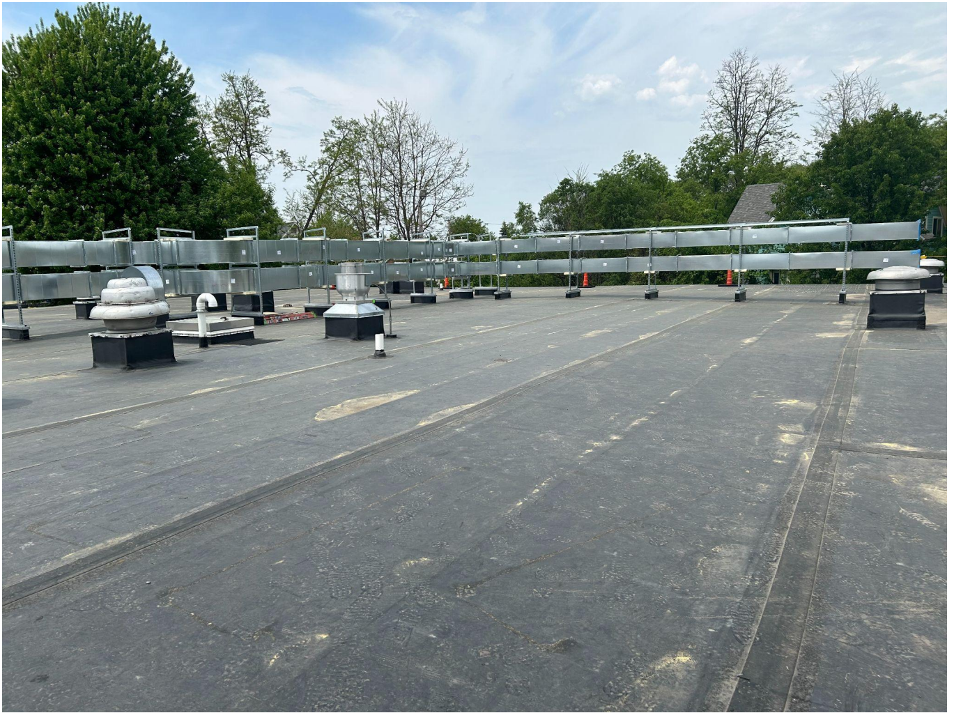
Second layer of ductwork added onto the roof supports for the 1965 wing.
