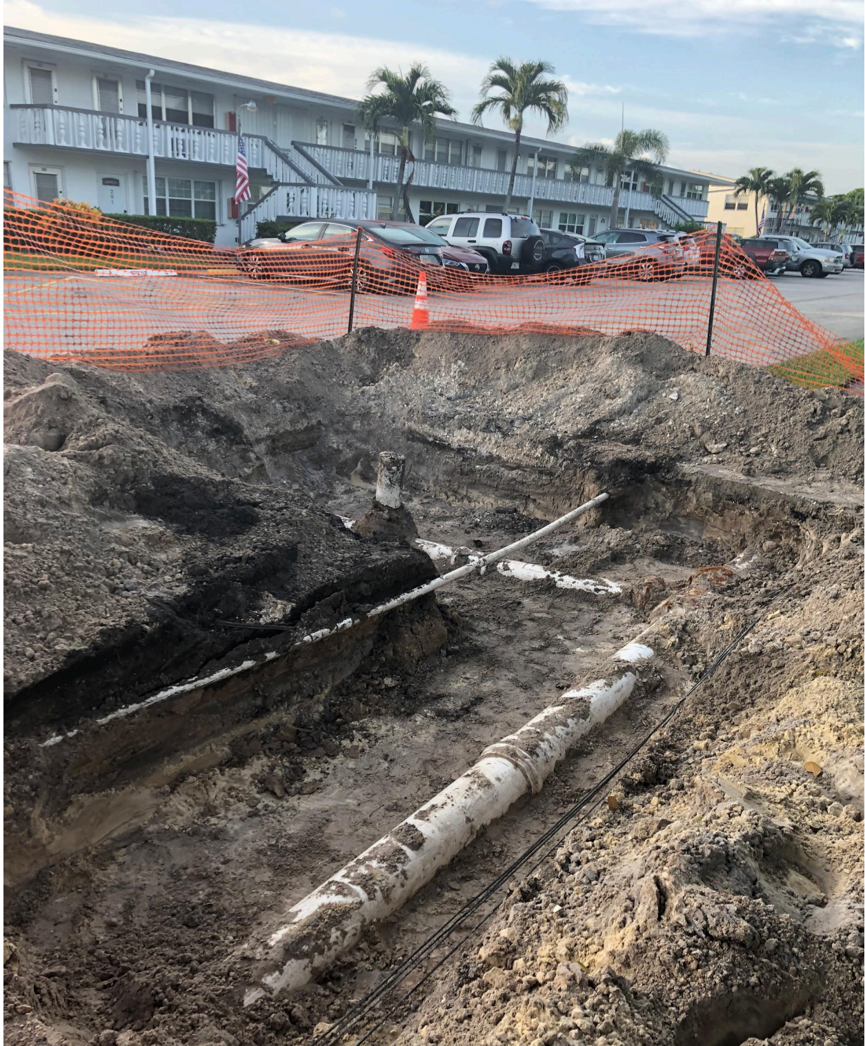
BERKSHIRE SECTION- THIS WATER MAIN PIPE SUPPLIES POTABLE WATER TO ALL OF BERKSHIRE SECTION. ADDITIONAL SHUT OFF VALVES WERE INSTALLED TO BETTER ISOLATE LEAKS.
