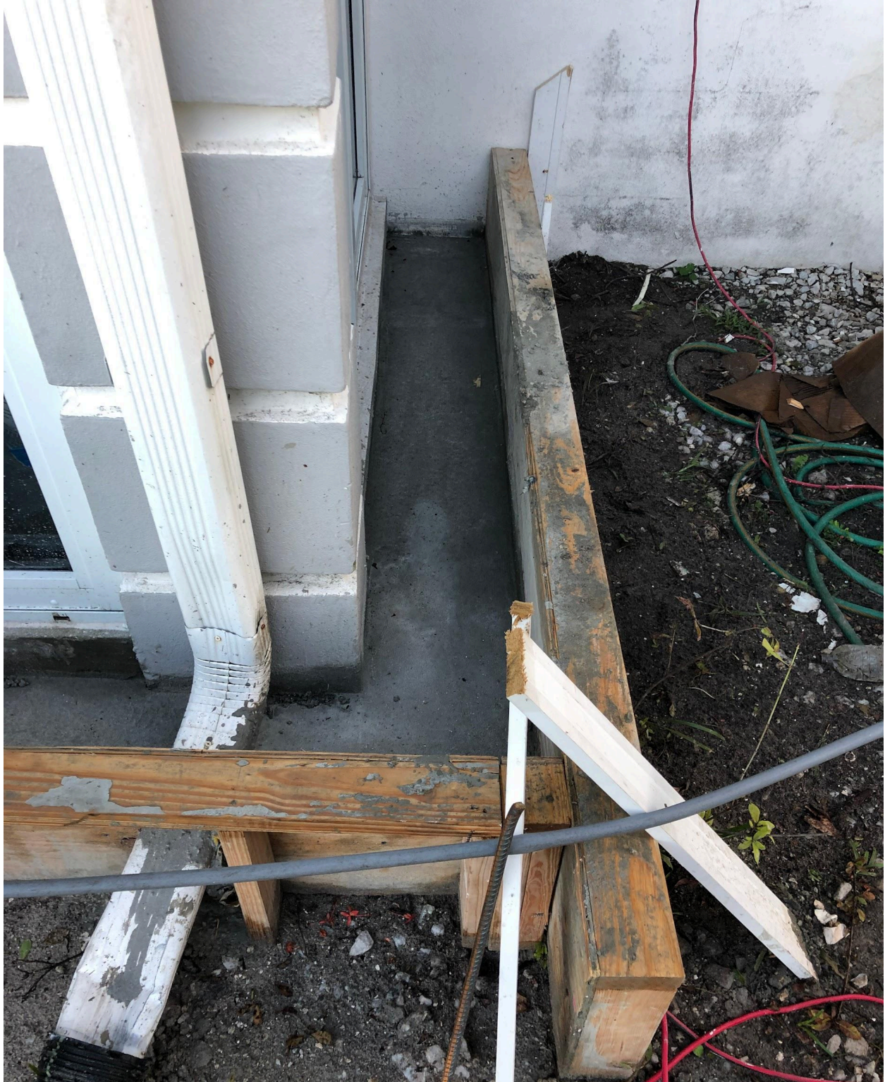
STRATFORD H- THE OWNER OF UNIT #97 HAD UNREINFORCED CONCRETE SLABS POURED AROUND THE OUTSIDE OF THE CORNER UNIT.
