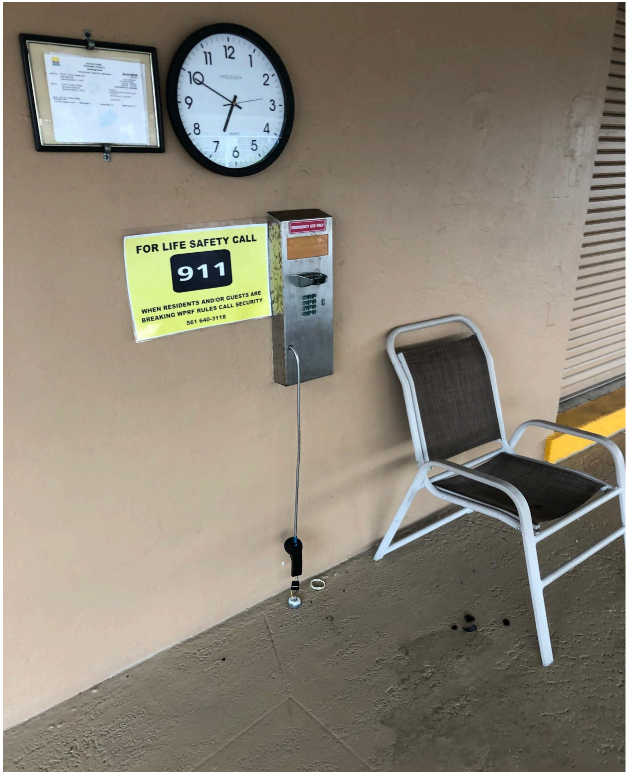
KENT POOL- EVIDENCE OF OVERNIGHT OCCUPANCY, AND VANDALISM, WERE DISCOVERED.
