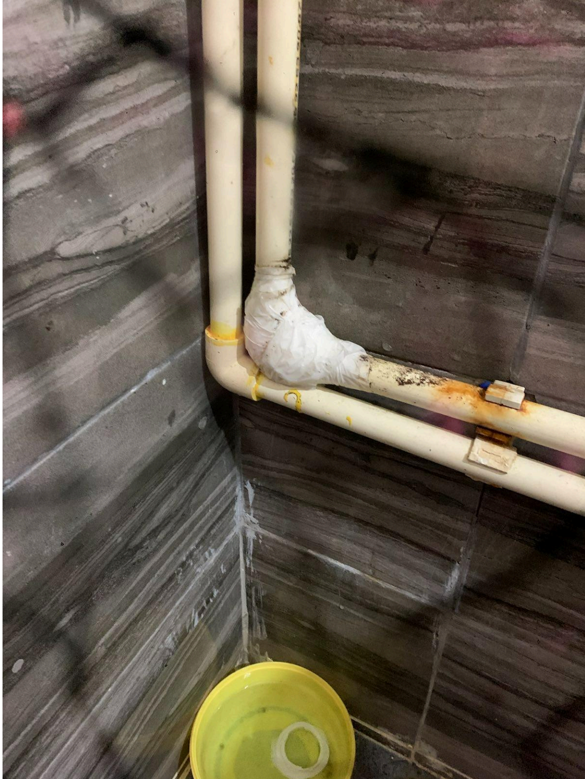
Extensive damage to plumbing in bathrooms; repairs made with what supplies the Khaya Family was able to access.
