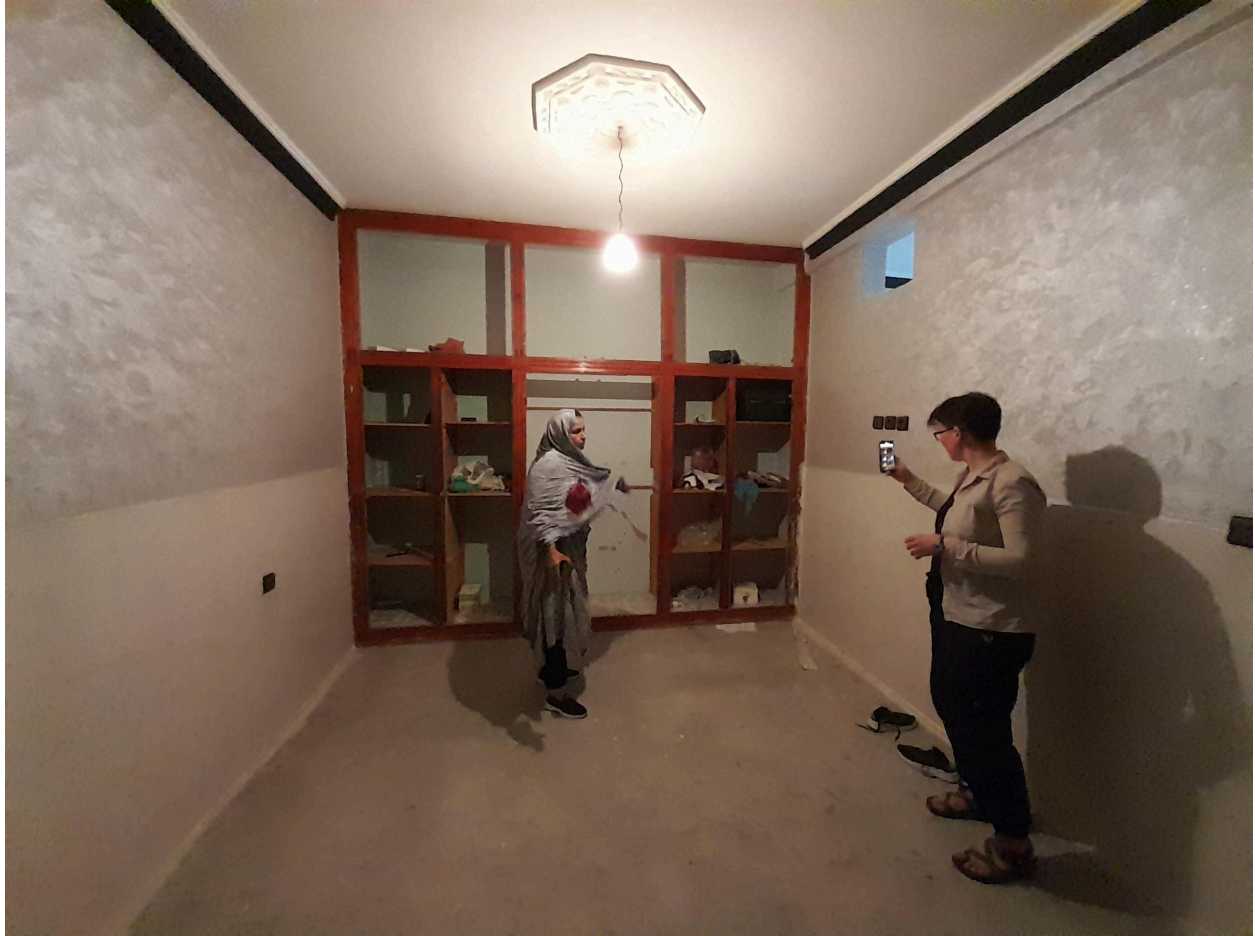
Cabinet doors were ripped off by Moroccan Occupation Forces during one of their raids on the home.
