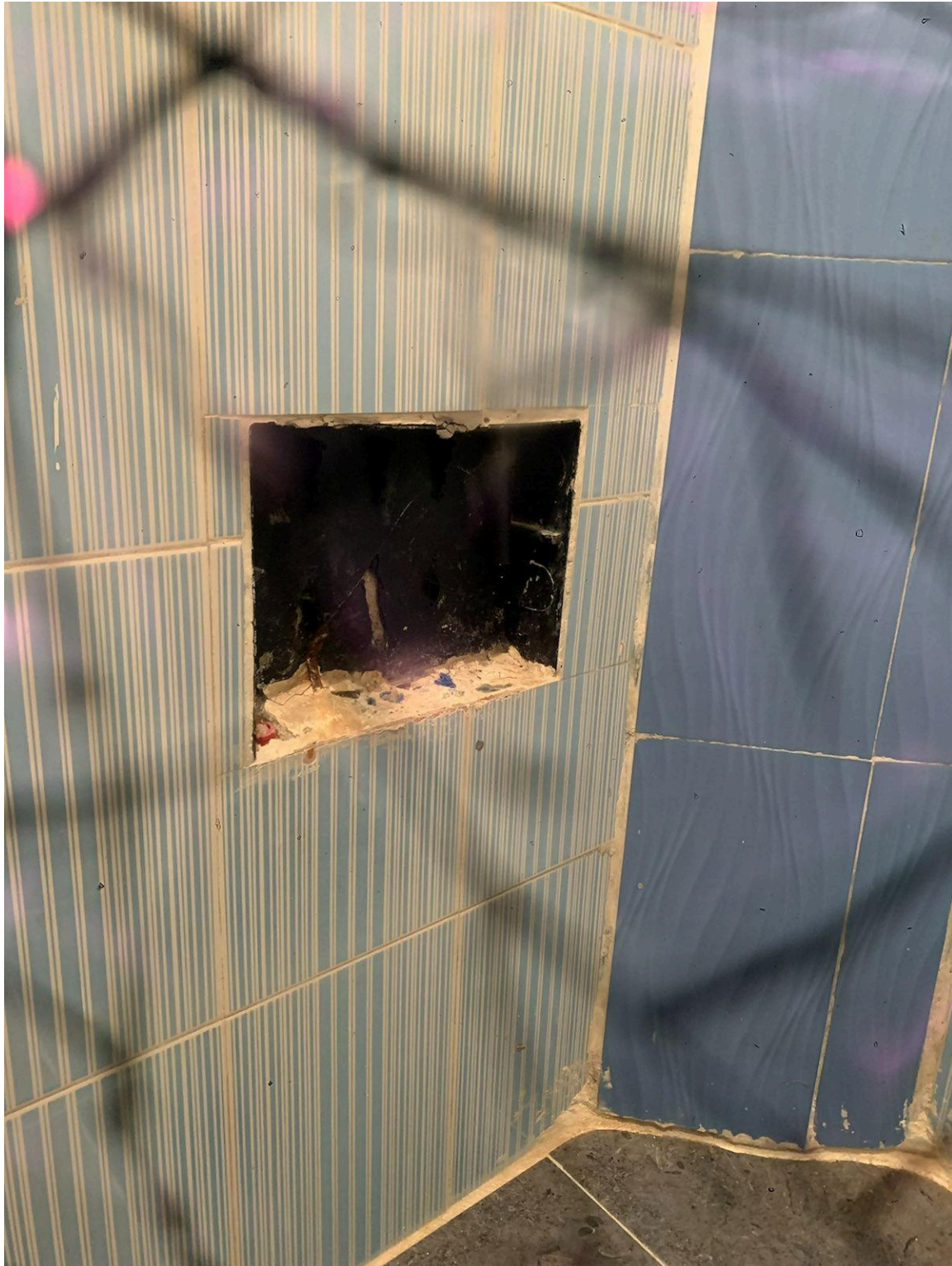
Bathroom cabinet ripped off of the wall.
