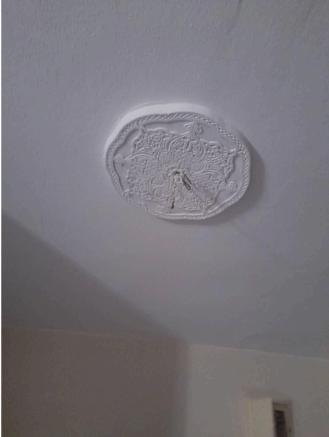
Lighting fixtures ripped out of the ceiling, seven fixtures were replaced over the course of the FV stay in the Khaya family home, Boujdour, Western Sahara.
