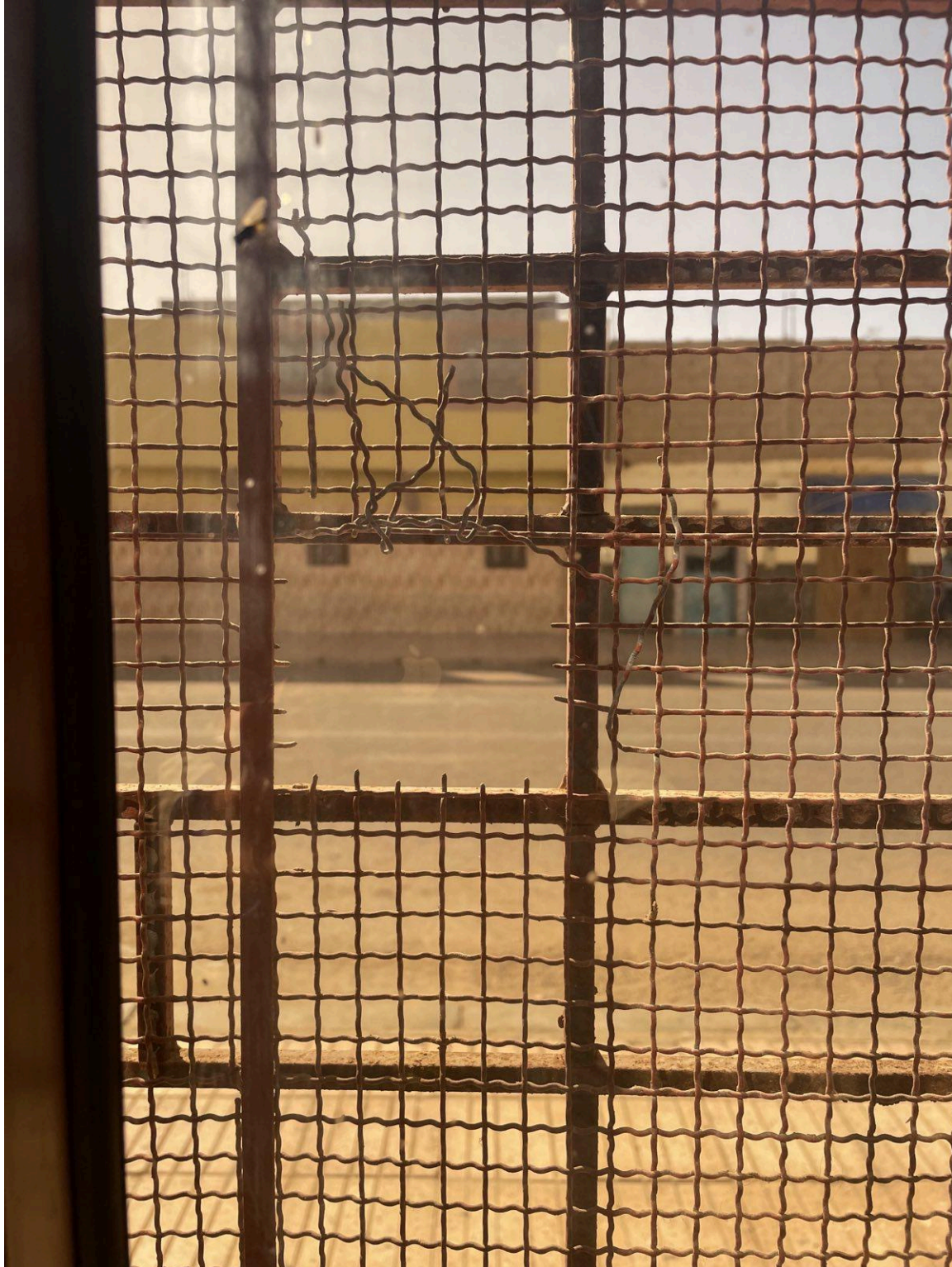
Damage to front windows of the Khaya Family Home in occupied Boujdour, Western Sahara.
