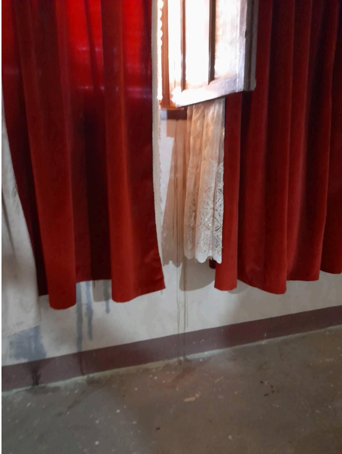
Stains on walls under windows, where chemicals were poured into the home.
