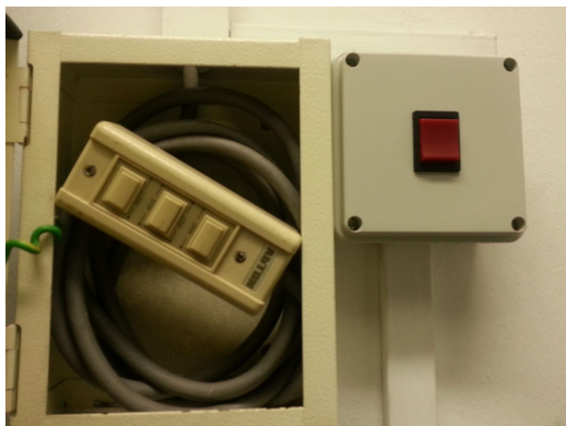
3) Left: Curtain switch Right: Screen switch
