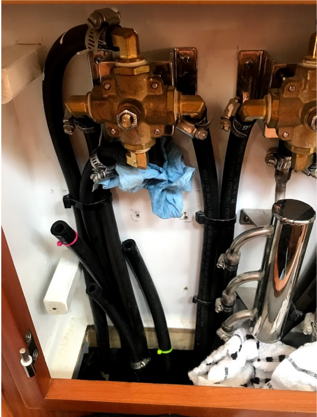
We removed the manifold and found debris in the elbow at the engine supply.
