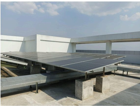
Example of Roof Mounted Solar Panels
