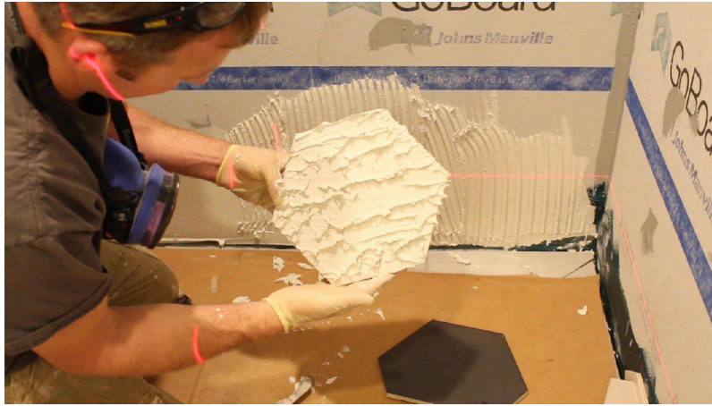
Pictured above: This tile has proper thin-set coverage.
