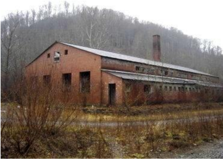
This dilapidated bath house is still in existence at Stonega. (Jan. 2007 image by author)
