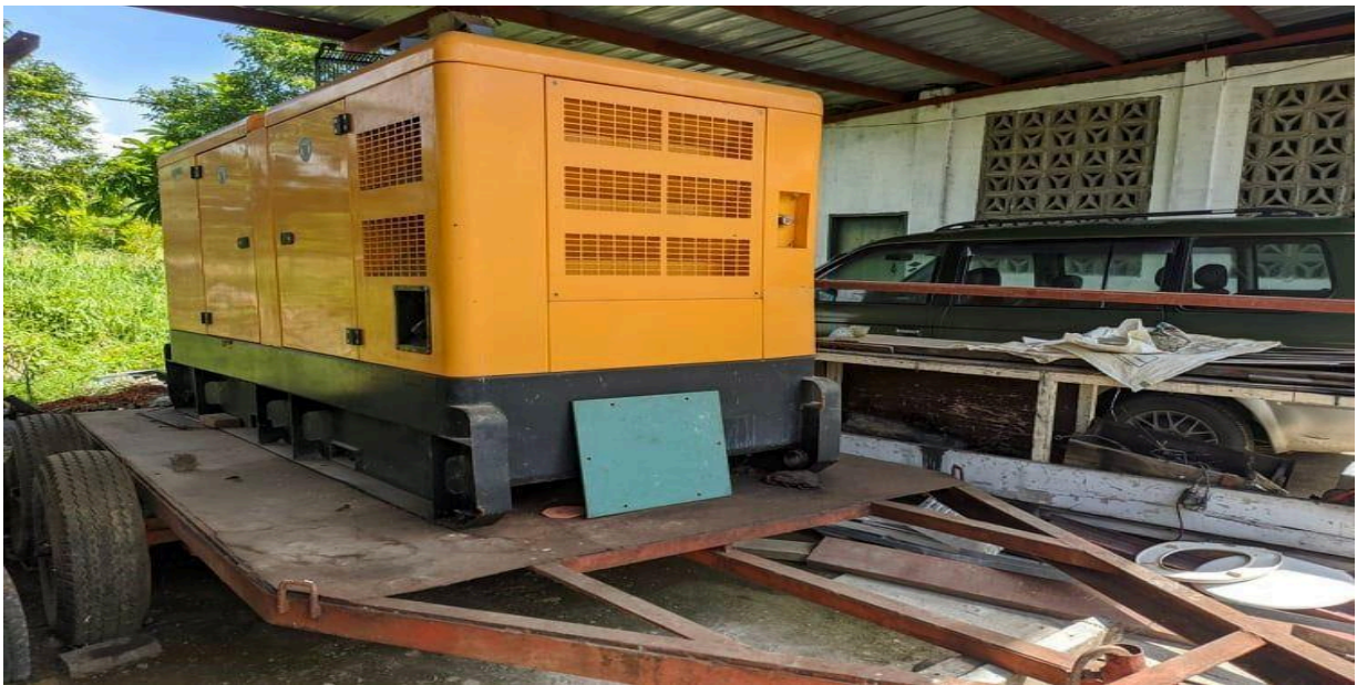
UNIVERSITY PORTABLE EMERGENCY POWER GENERATOR
