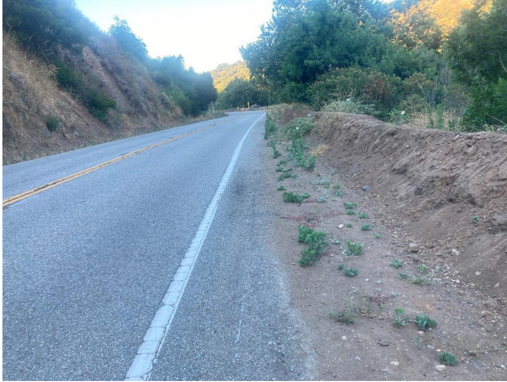
Figure 9: Glendora Mountain Road facing south showing berm on side of road, July 29, 2024.
