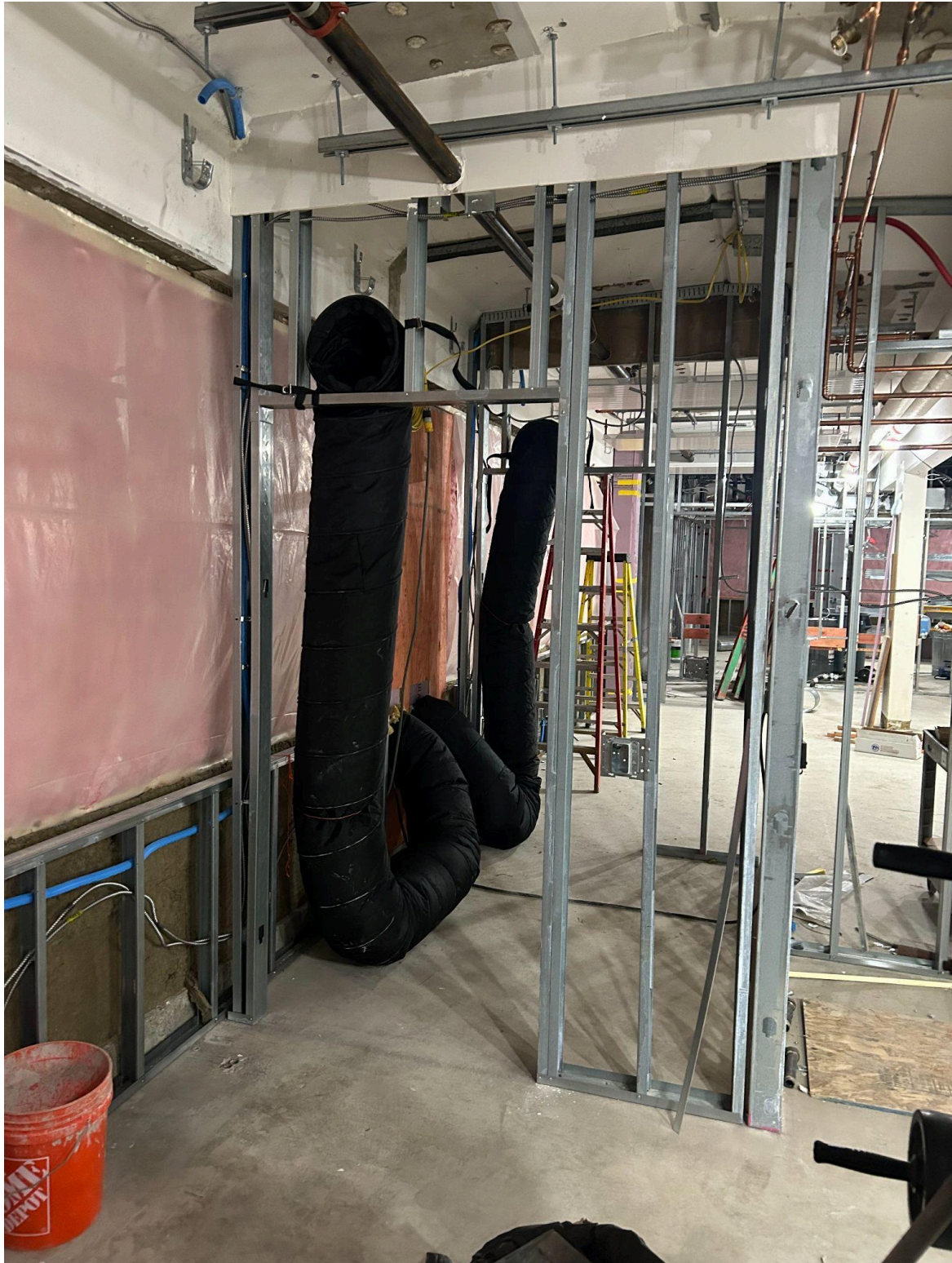
The tubes from the temporary heater come into the building and terminate with these flexible ducts blowing the warm air into the 1965 wing of the building.
