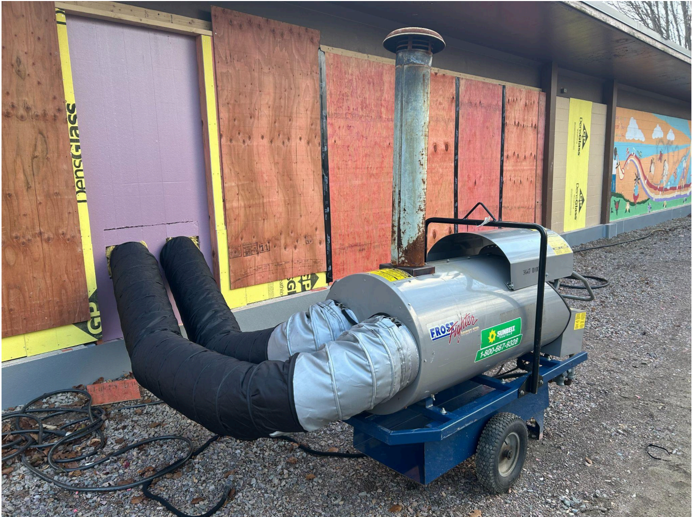
A picture showing a gas fired heater that the contractor has installed as a temporary measure to help with the heating of the building in the 1965 wing.
