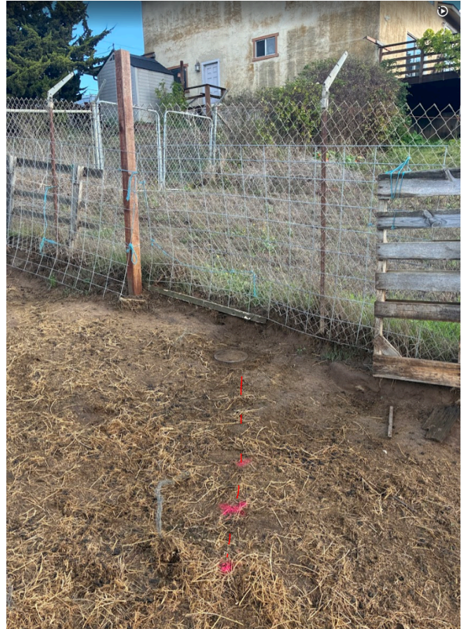
PVC line where riser broke -- and it's been capped, but it is not controlled by shut off on 4 Bayview. Controlled by one of the 2 on Elkhorn Road
