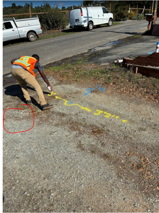
7'+ under the secondary driveway on the right side. Side. so deep the signal was dropped.
