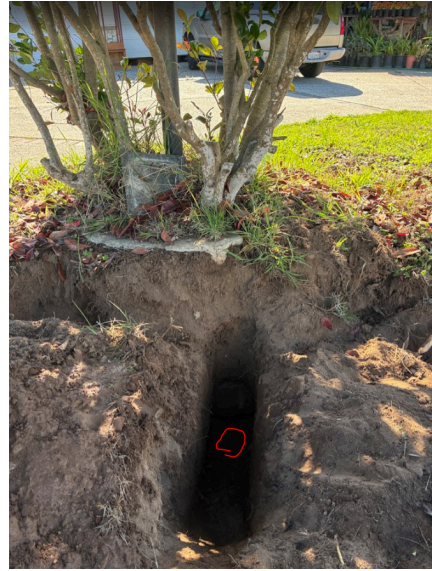
The T for the mainline was found about 22" below grade right under edge of ring around tree
