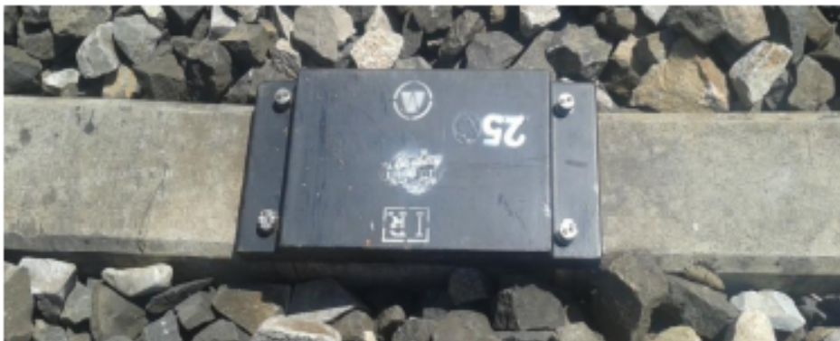
RFID Tag fixed on sleeper
