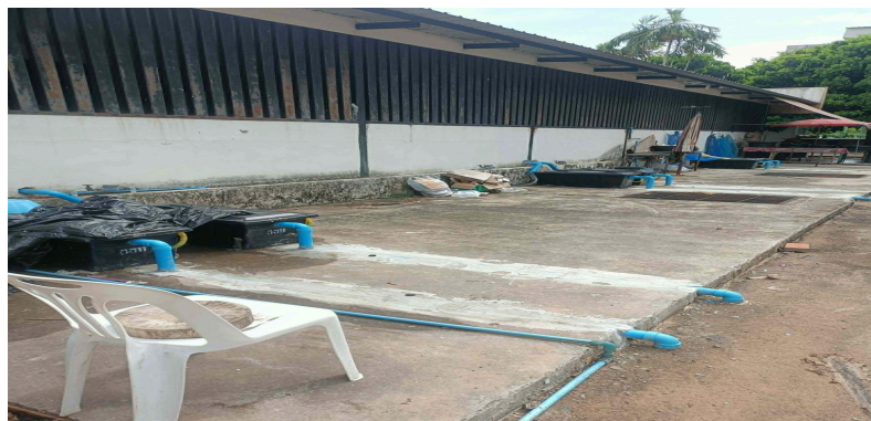
Grease Trap and Microbial Wastewater Treatment System
