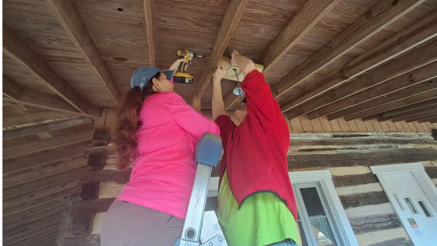
Photo by Tysha Robinson: Pictured: Ellen Feer, JT Tucker - Installing ceiling fans on the porch
