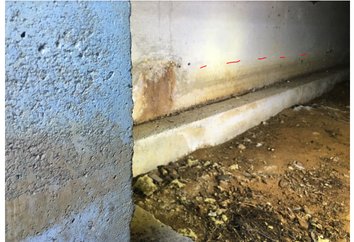
12" high water line
