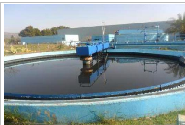
Figure 4a. Final clarification basin.
