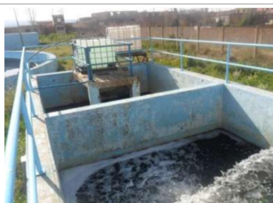
Figure 4b. Post chlorination basin.
