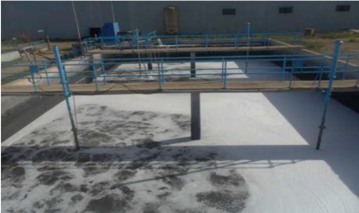
Figure 2. Photo of mixing and equalization basin N ° 1.
