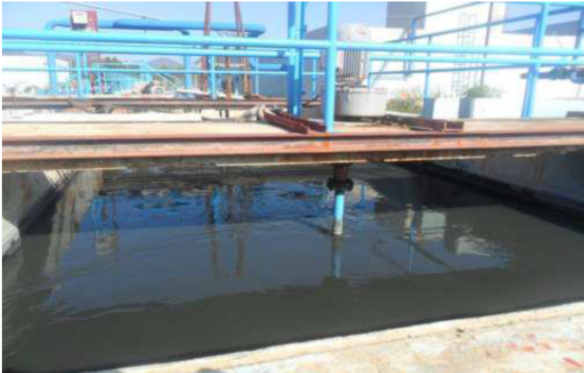
Figure 3. Mixing and neutralization basin N ° 2.
