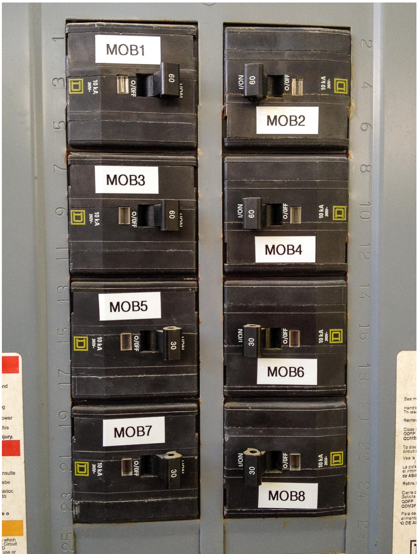
Circuit Breaker Panel B (outside panel) close-up. The Master key “MK” opens the lock for this panel.
