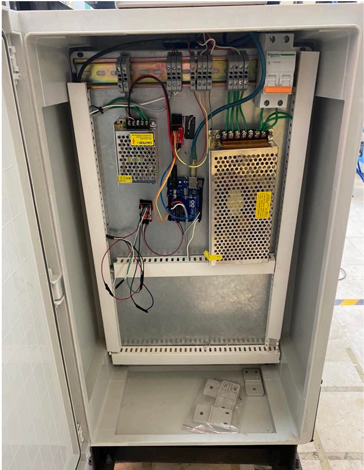
Figure 3-3: control board of Savinoux turbine
