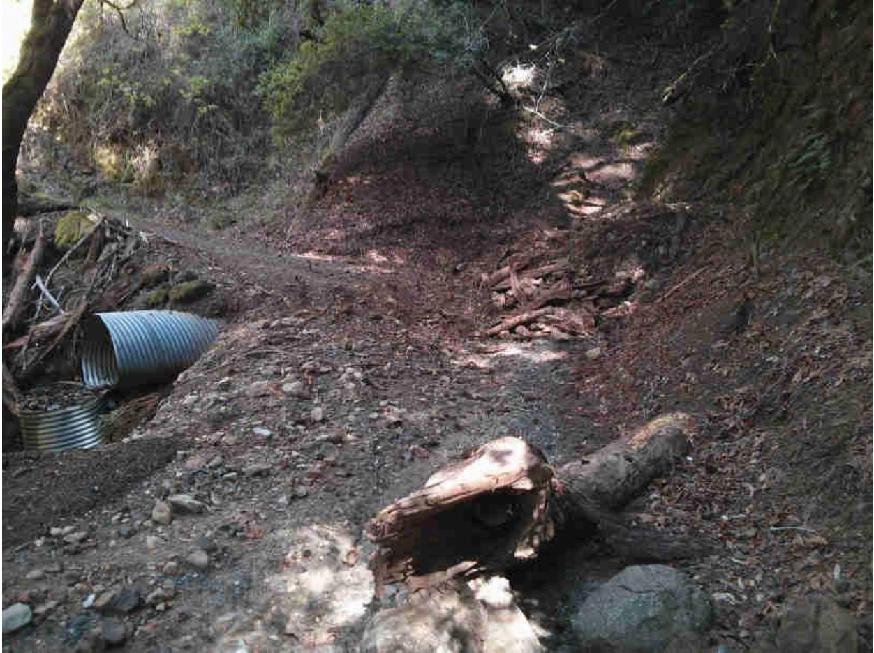
Fig. 8. School Rd culvert damaged suffered during February, 2015 rainstorm
