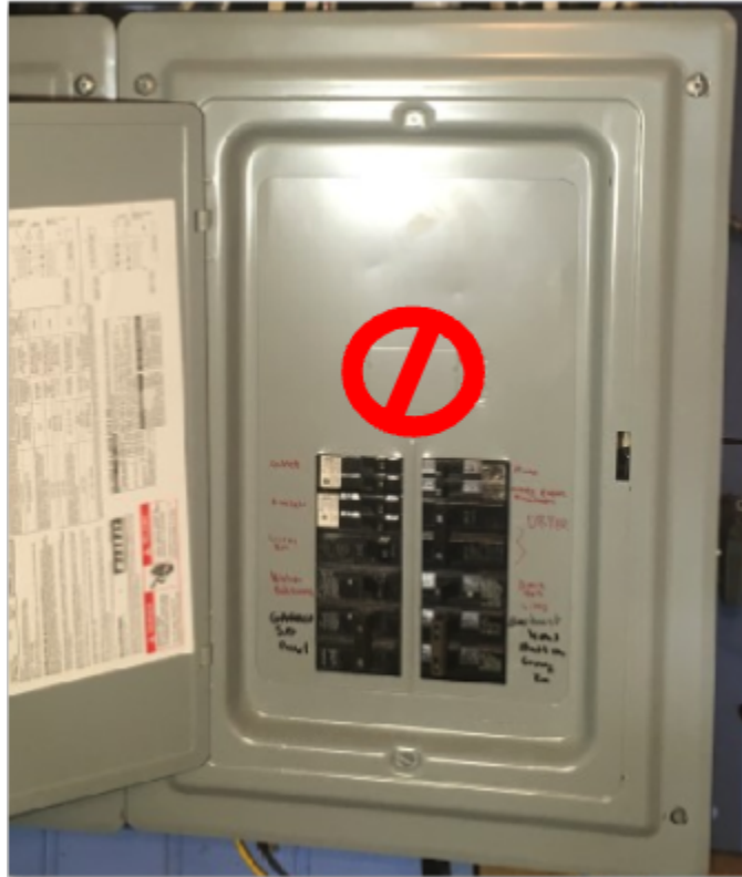
No Main Breaker
