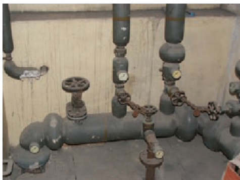
Old heating system containing brown, white and blue asbestos - some damage
