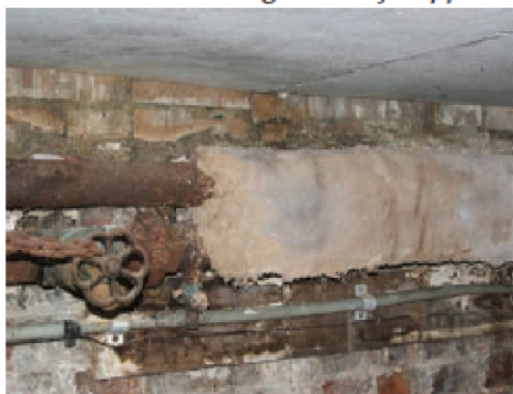
Damaged asbestos pipe insulation
