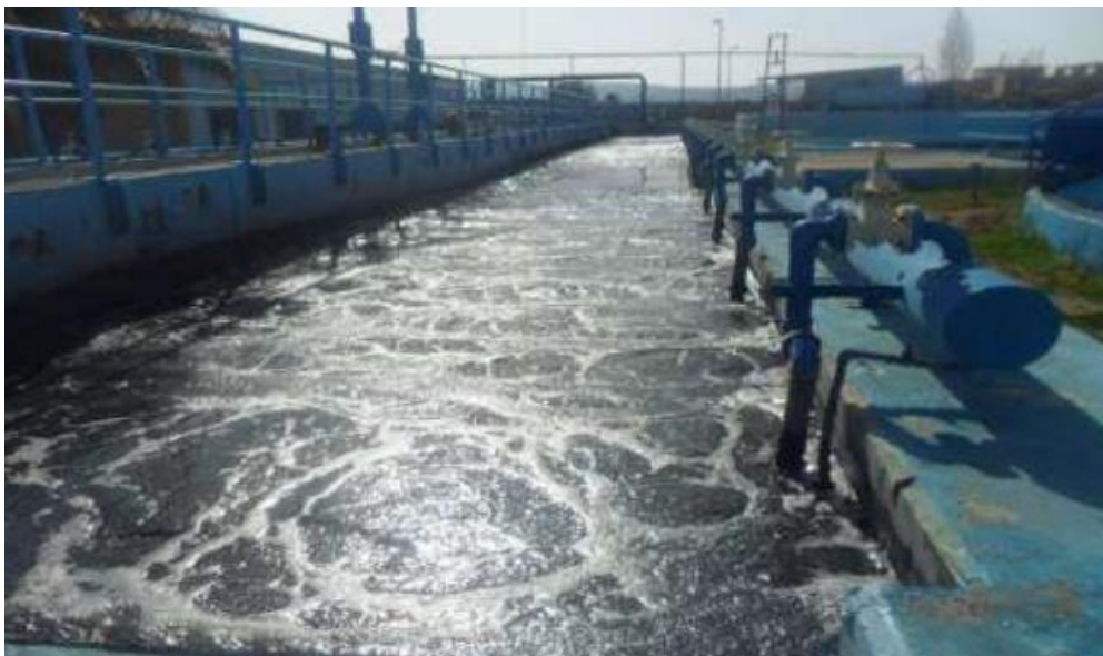
Figure 5. Biological basin (aeration basin).
