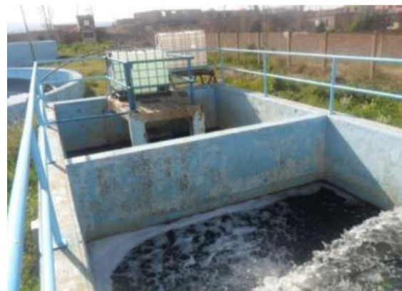
Figure 6b. Post chlorination basin.
