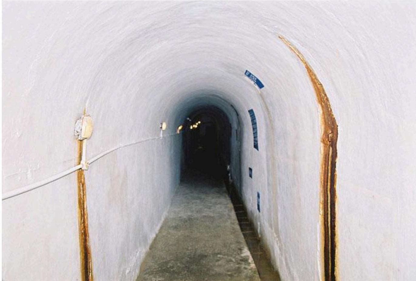
Inside view of gallery. There is not enough oxygen to breath inside this gallery.
