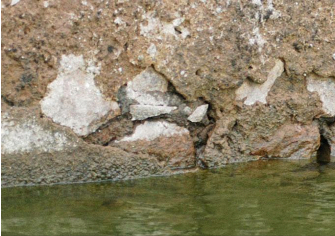
Cracks on the main wall. and the water is entering into the dam.
