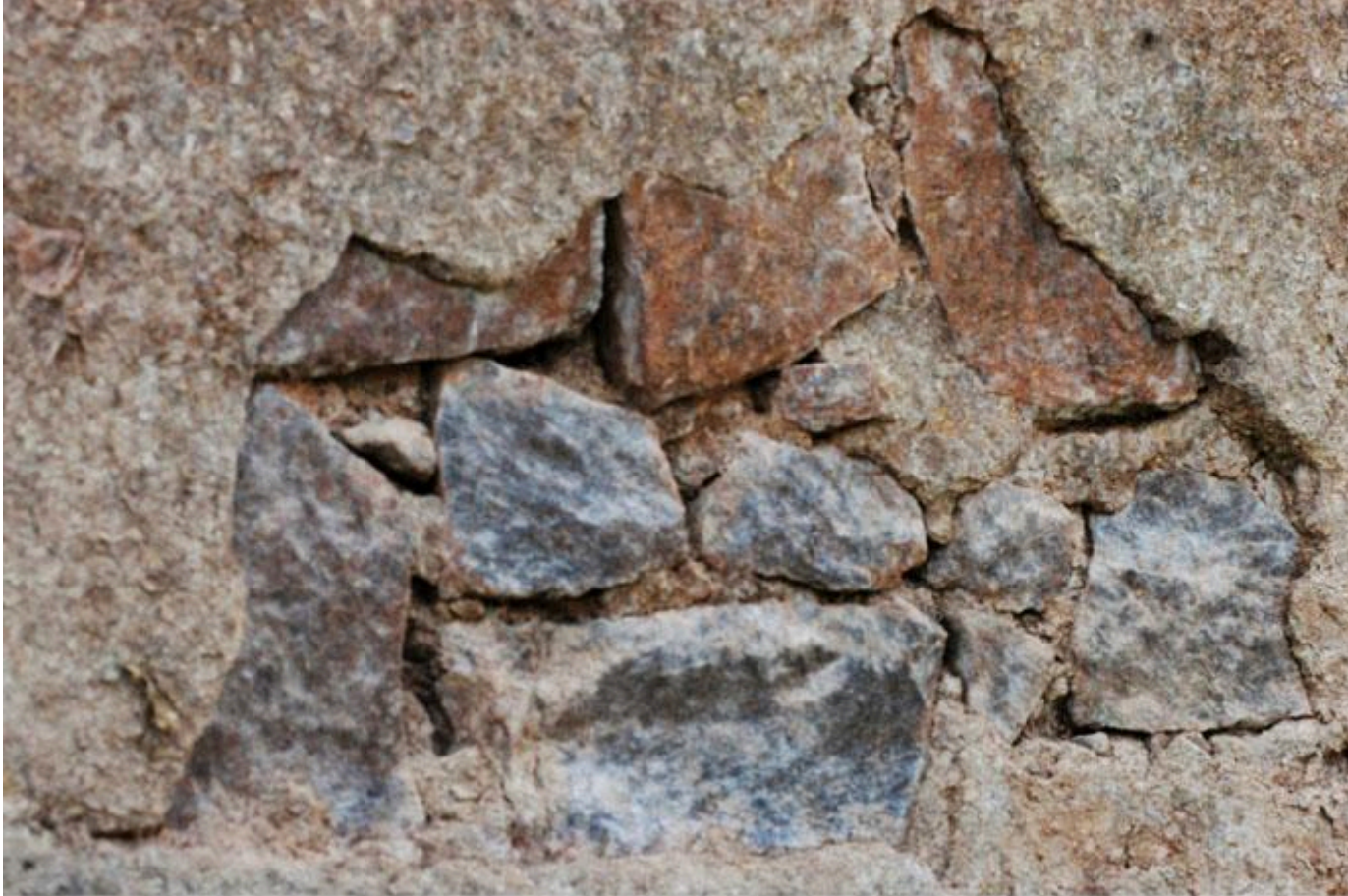
The plaster is gone. Only stones leave. A dam on Bare Stones.
