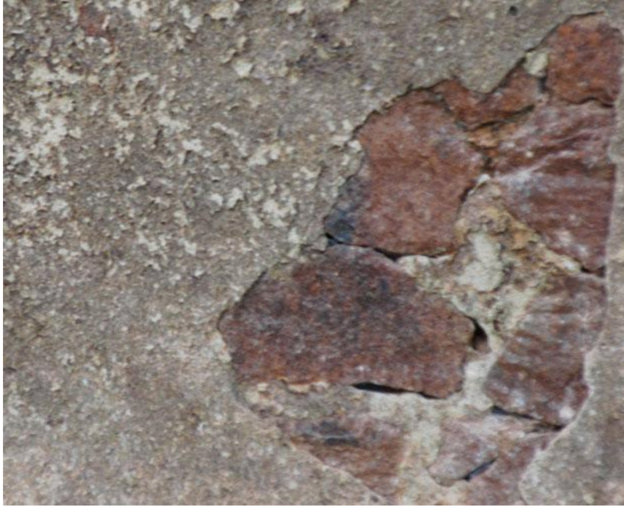
No Plasters in between the stones.
