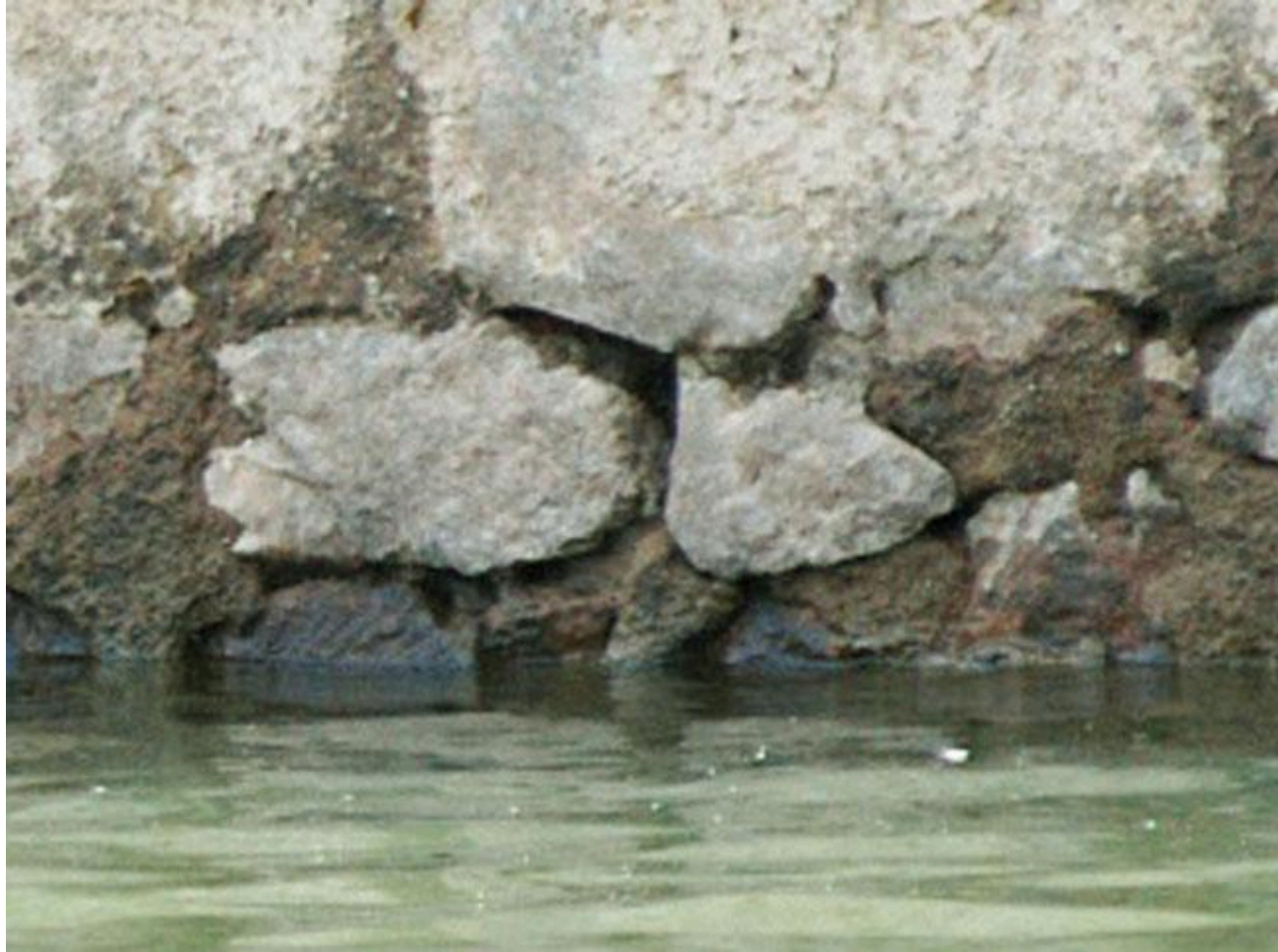
Cracks Cracks on the wall...
