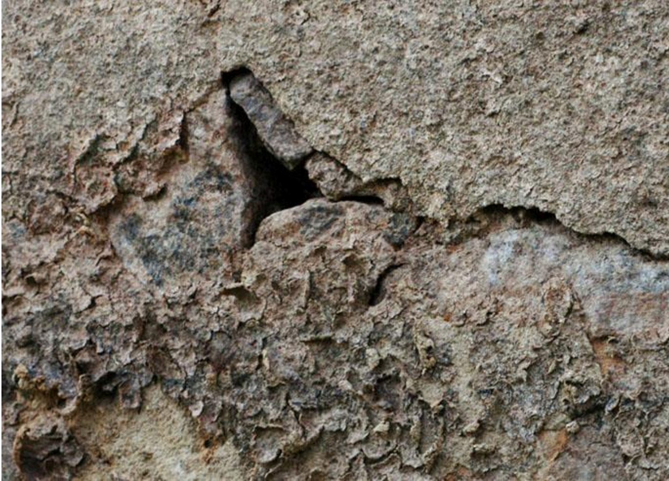
Cracks between the stones.
