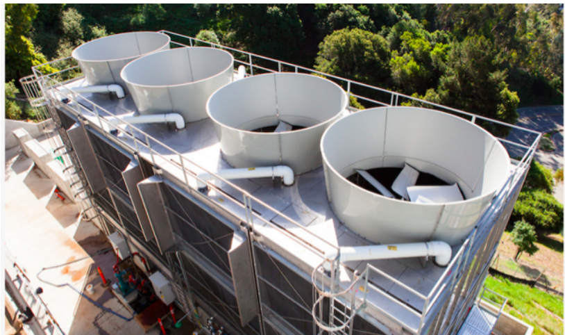
Cooling towers at Shyh Wang Hall reject heat from the high-performance computing center.
