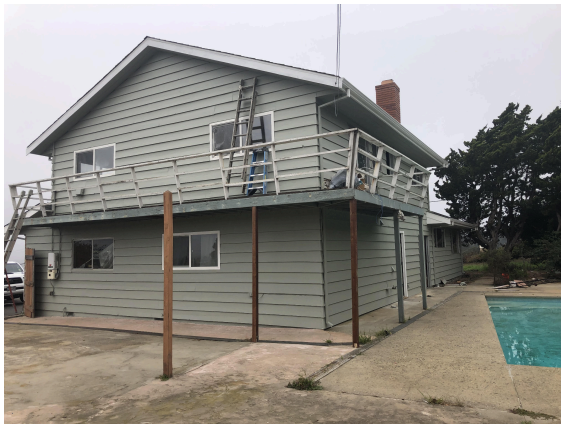
Home with the defective deck during preparation for sale in September 2020.
