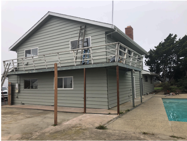
With structurally unsound deck in September 2020, during prep for sale
