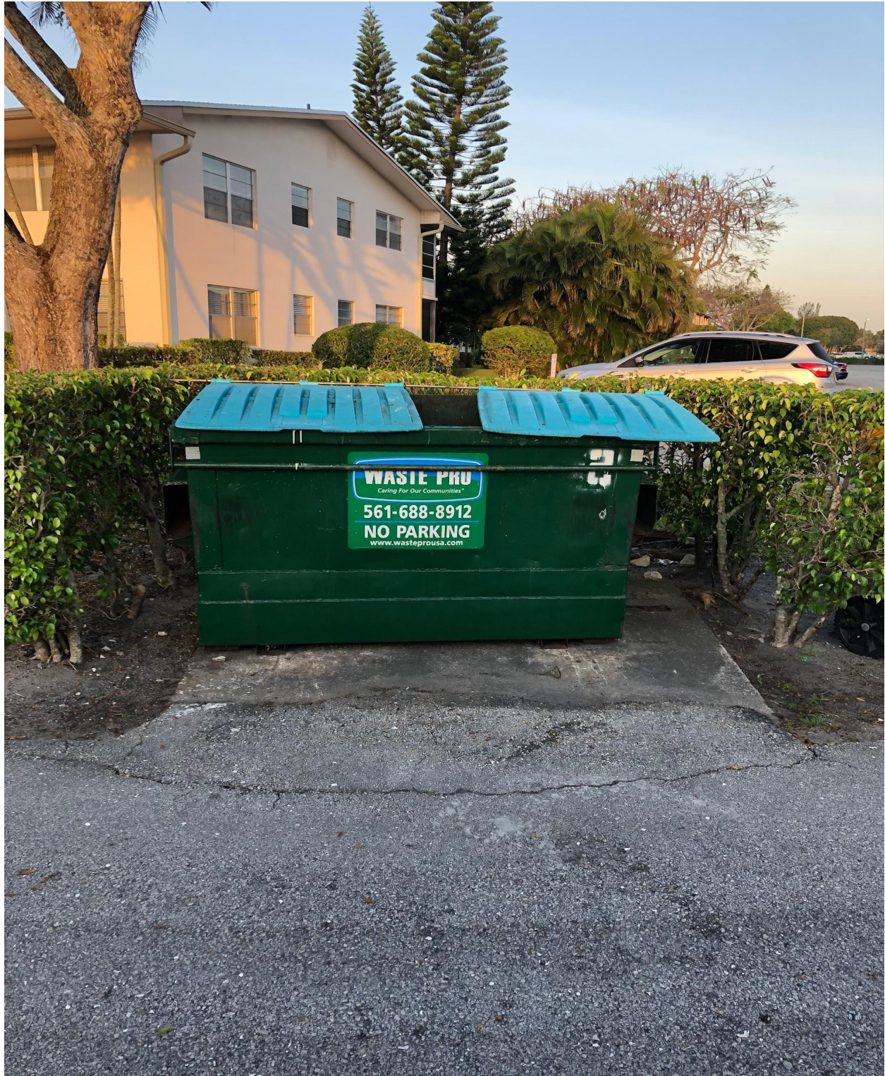
KENT H- DUMPSTER WITH BUSTED LID. REQUEST FOR REPAIR WAS SENT TO WASTE PRO.
