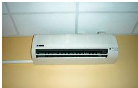
Gambar 1. Air Conditioning (AC ) secara umum
