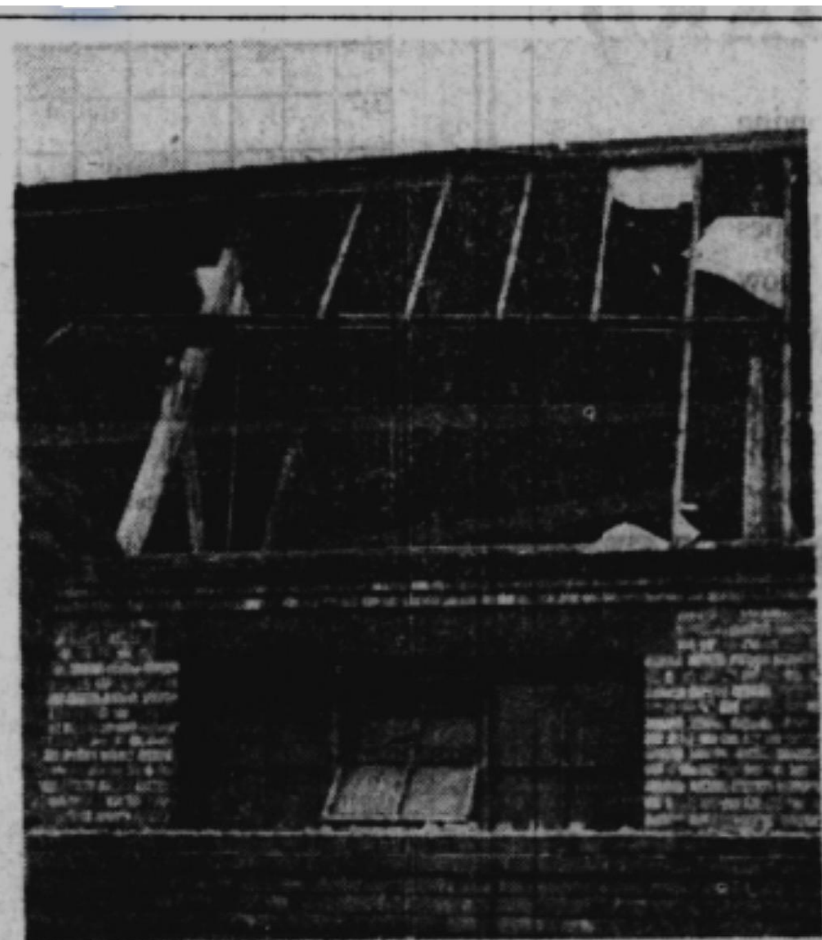
Birmingham Gazette photograph. Roof of the Serck Radiator Company's premises in Warwick-road, Greet, bared by the force of the terrific gale.
