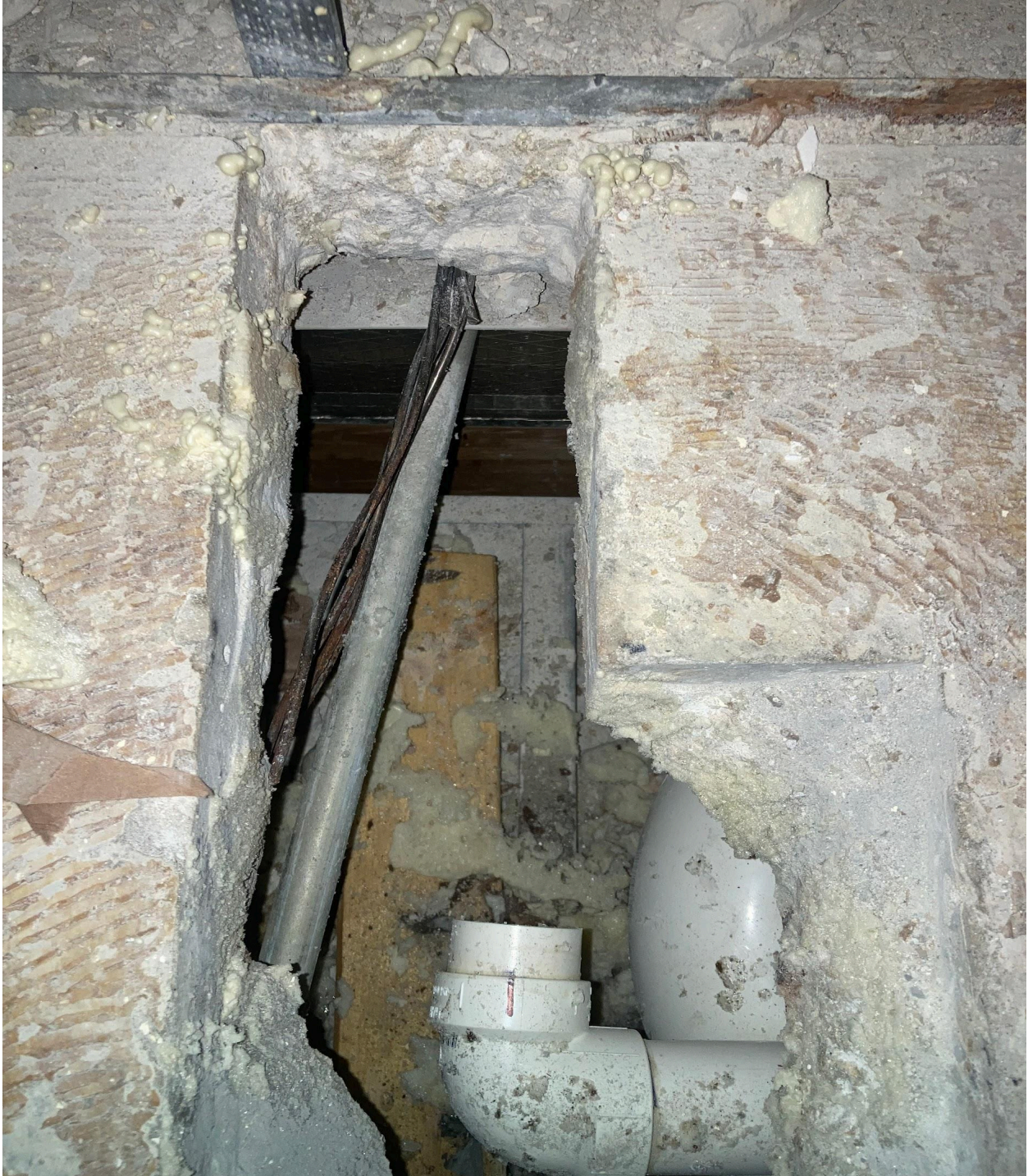
WELLINGTON L- THE OWNER OF UNIT 305 JACKHAMMERED STRAIGHT THROUGH THE FLOOR TO THE UNIT BELOW.
