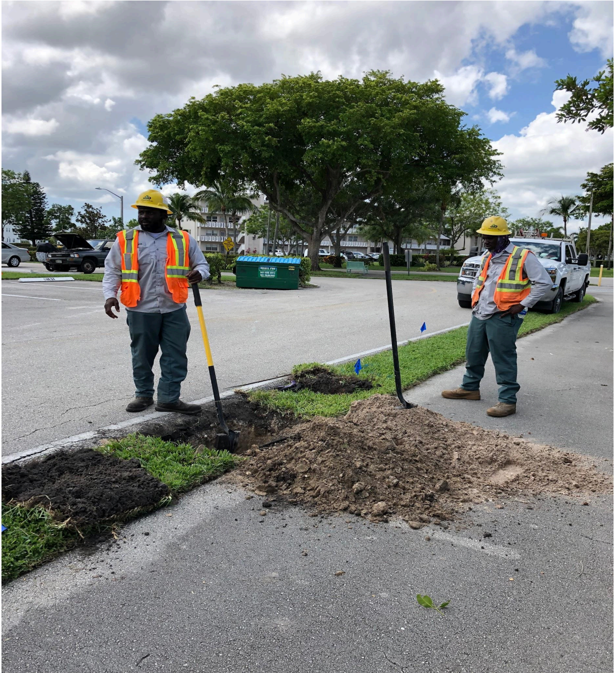
BERKSHIRE SECTION- JOHNSON & DAVIS CONSTRUCTION HAS RESUMED INSTALLATION OF POTABLE WATER VALVES AT VARIOUS SECTIONS OF CV.
