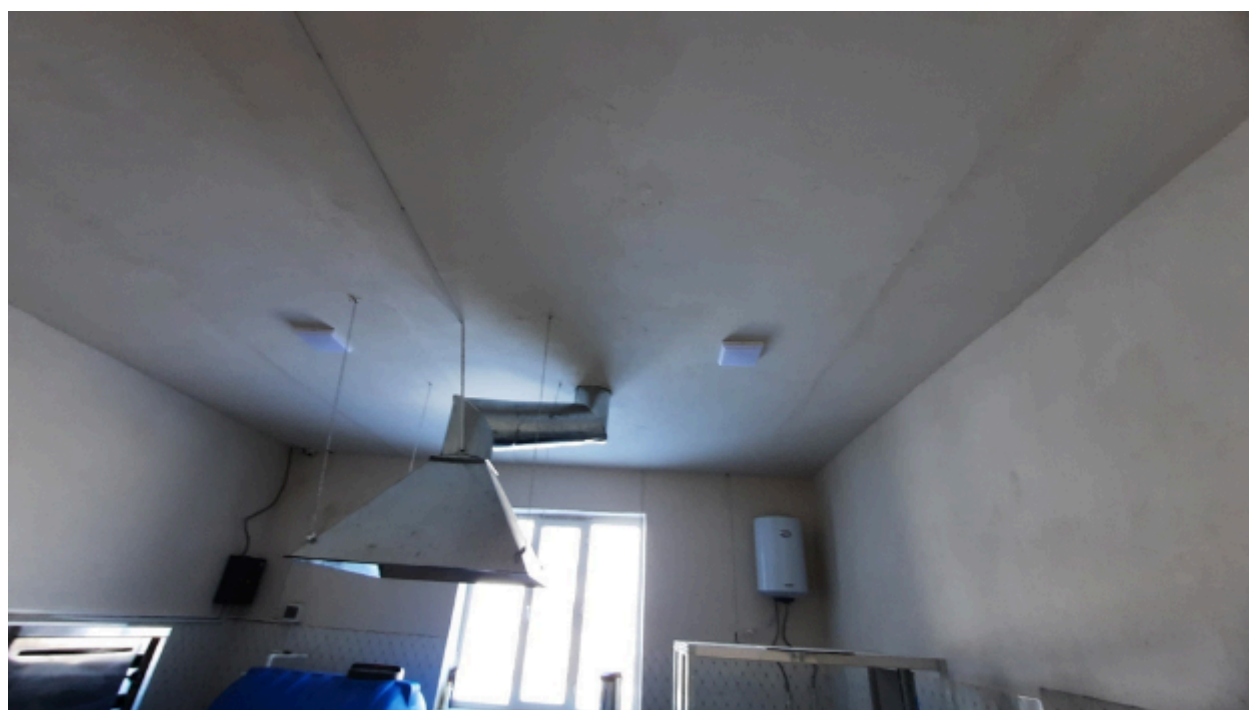
Photo 9. Local ventilation exhaust in block No. 1-3 in the kitchen
