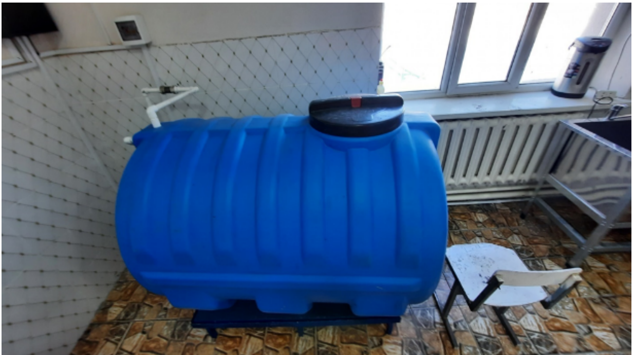
Photo 13. Water tank for the canteen needs
