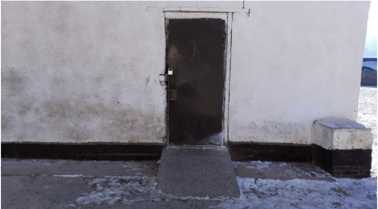
Photo 18. Building No. 2 has a ramp, but it does not meet the requirements.
