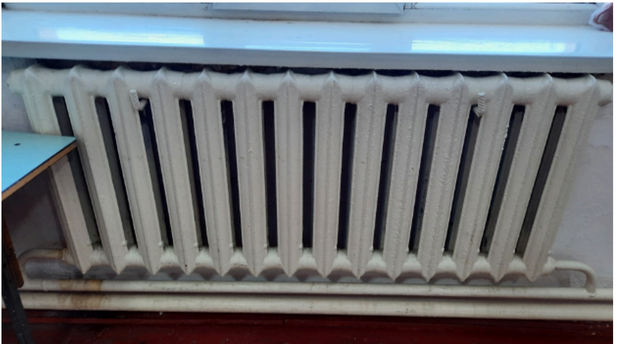
Photo 7. Type of cast iron radiators installed
