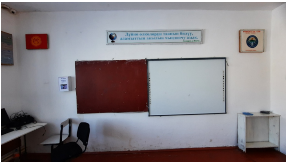
Photo 8. There are no ventilation shafts or air ducts in the classrooms.
