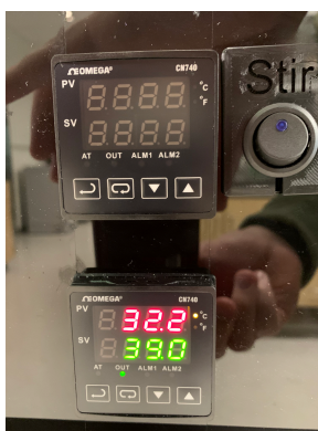
Fig. C4. Powering up the MRM Temperature Controller.
